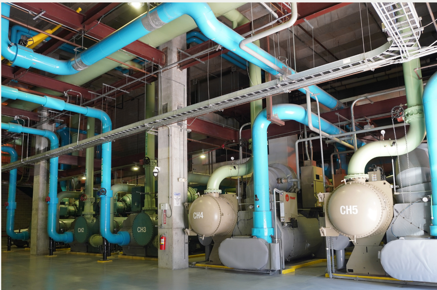
Inside the CentTrio District Cooling facility
